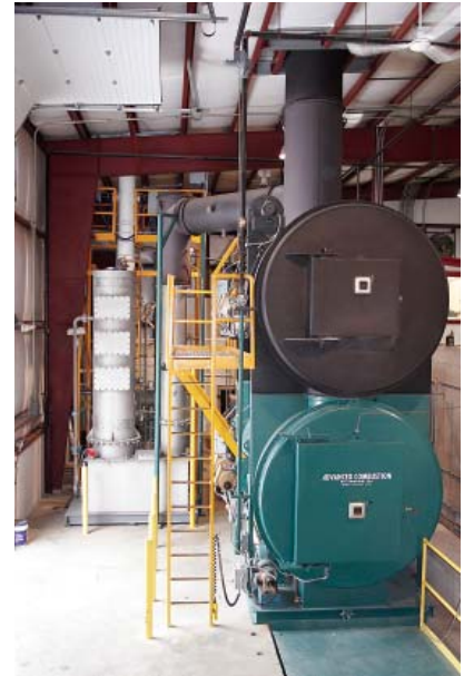
ACS MSW Incineration System with Scrubber
